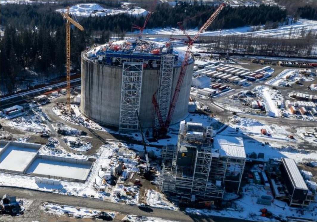
PHOTO 5: LNG STORAGE TANK AND BOIL OFF GAS AREA (MARCH 2023)
