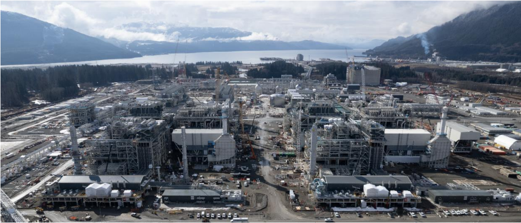
PHOTO 3: LNG FACILITY – VIEW FROM LNG TRAINS TO THE SOUTH (APRIL 02, 2023)
